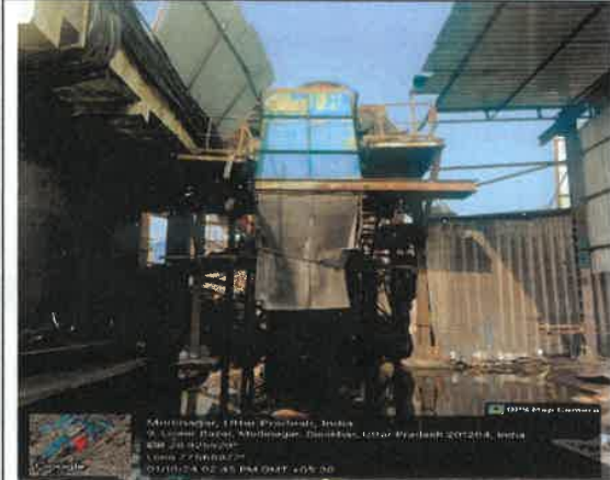
Loading platform of wet fly ash after clarifier.
